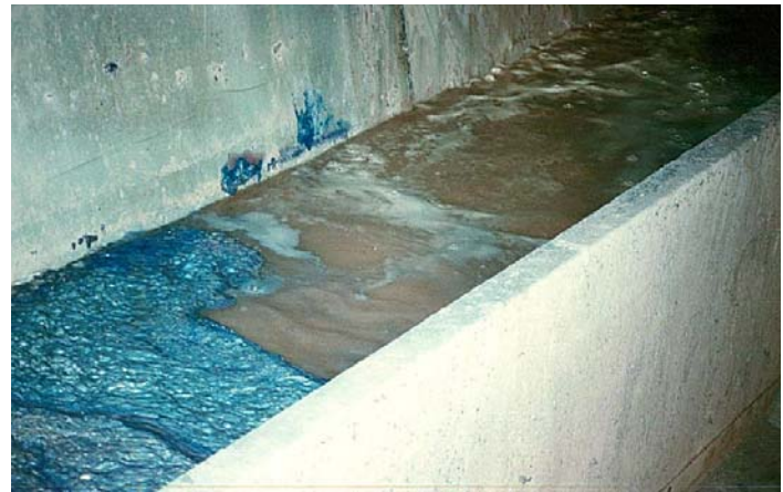
Water Wash Booth with Paint Contaminant
